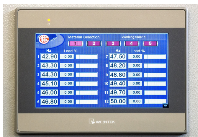
Figure 2: Control panel of the rolling mill with variable speed
